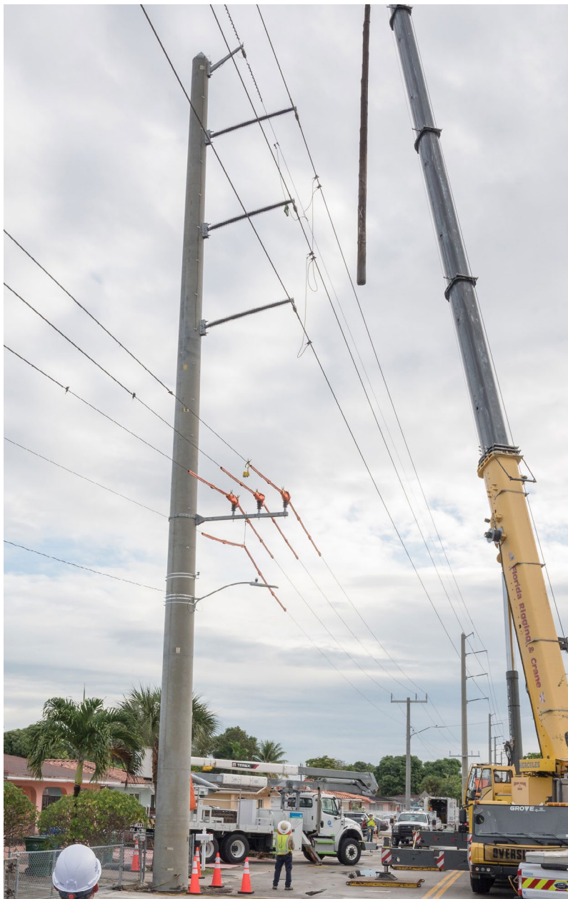
FPL has replaced nearly all of its wooden transmission poles across its service area with concrete or steel poles.
