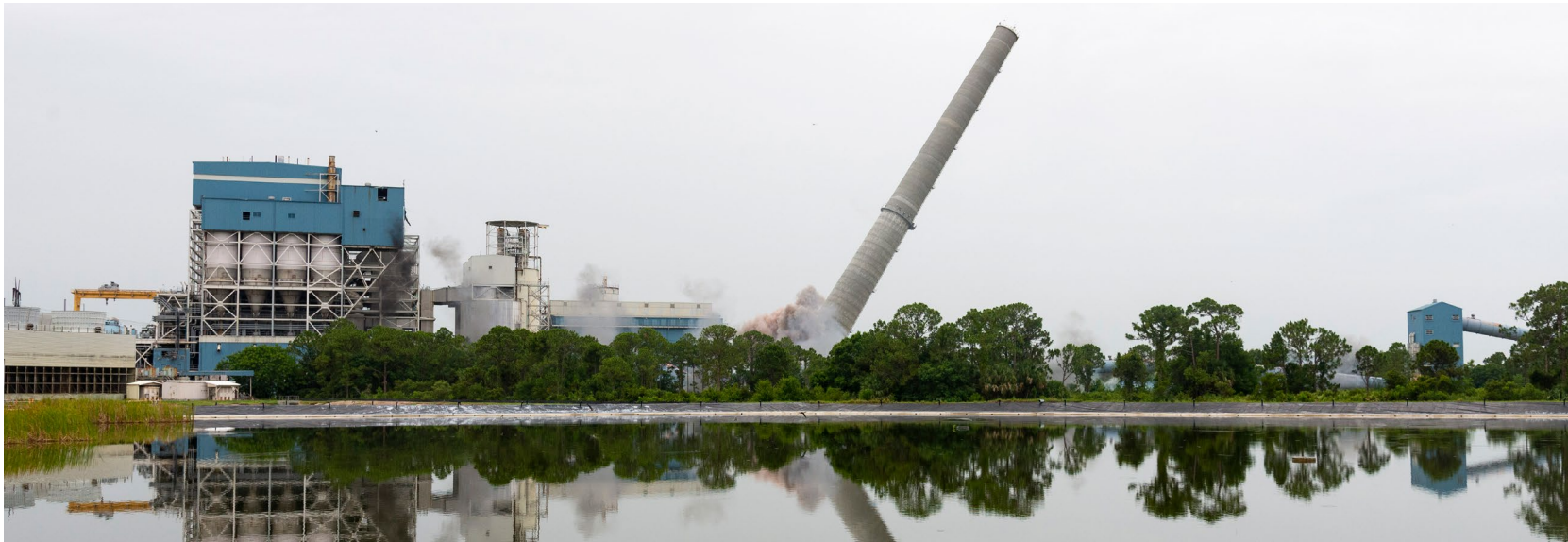
A tower at the Indiantown Cogeneration Plant in Florida is captured mid-collapse during its implosion.
