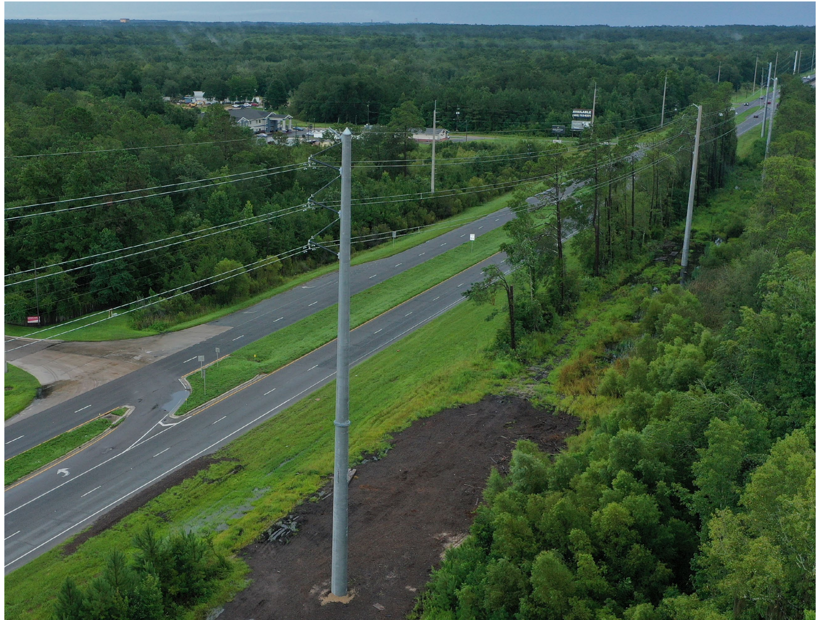
North Florida Resiliency Connection transmission line connects FPL's Northwest Florida customers to the larger energy grid that serves FPL customers throughout the rest of Florida.
