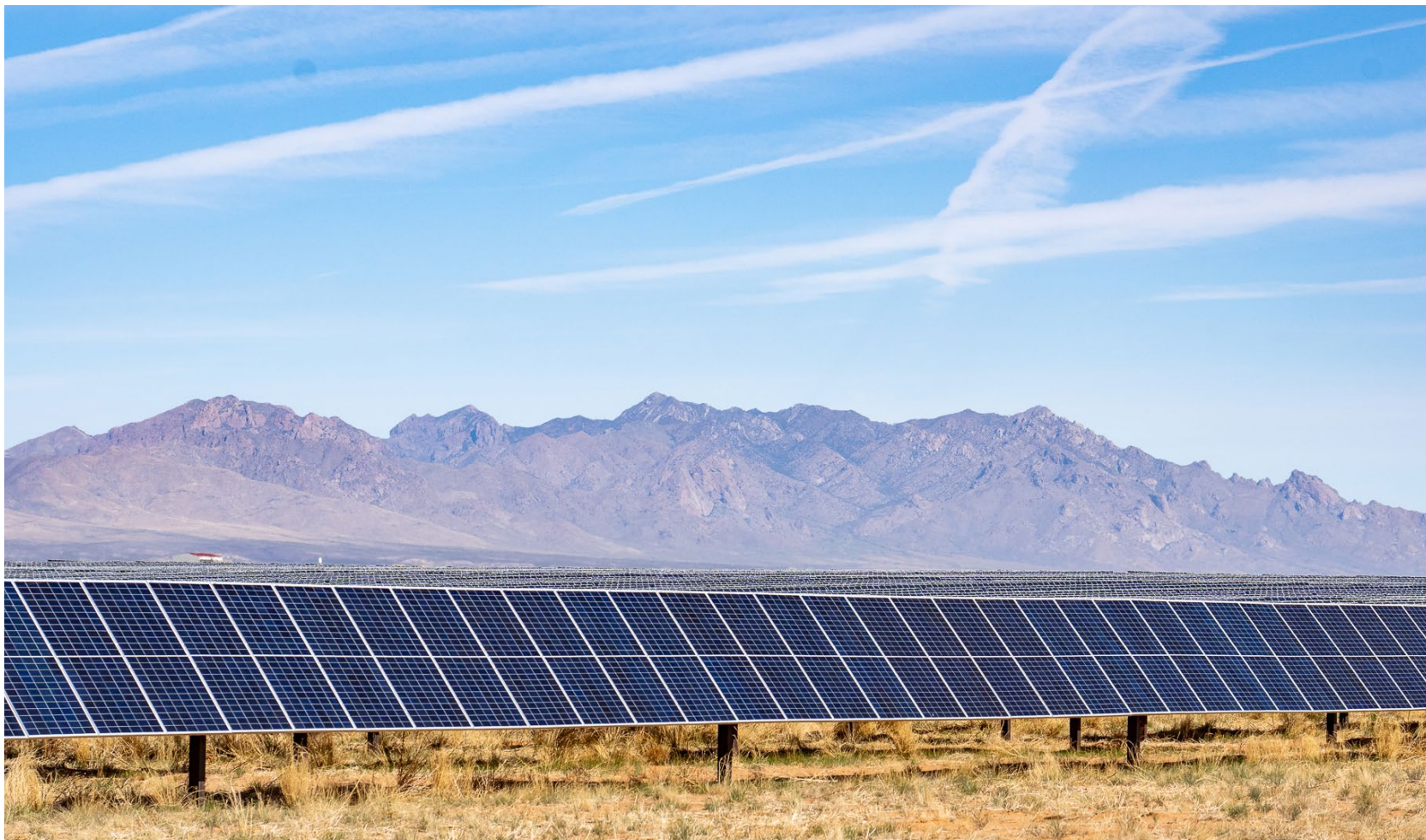
The Buena Vista Energy Center in Chaparral, N.M.
